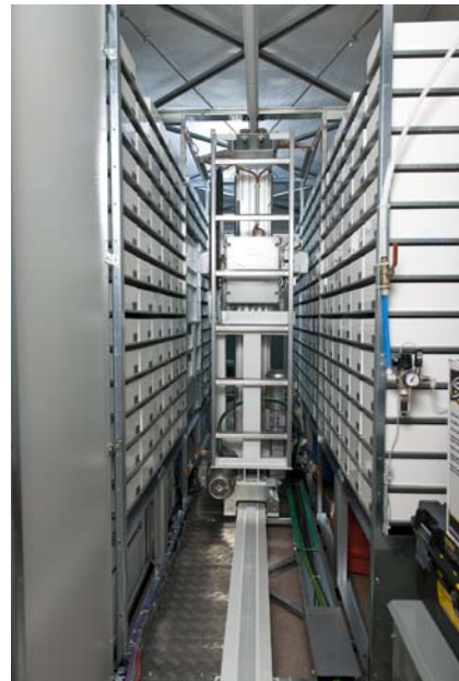
Photo Caption: An inside shot of the Swisslog Boxpicker that was installed at OTMH June 2012.
